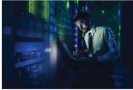
Data Center Rooms
