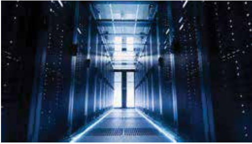
Rooms Requiring Precision Cooling
